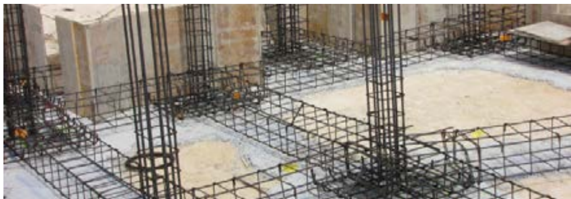
Forjado sanitario sobre muro de fábrica de hormigón cimentado sobre zapatas y vigas. Foundation structure is composed by footings and foundation beams from reinforced concrete.
